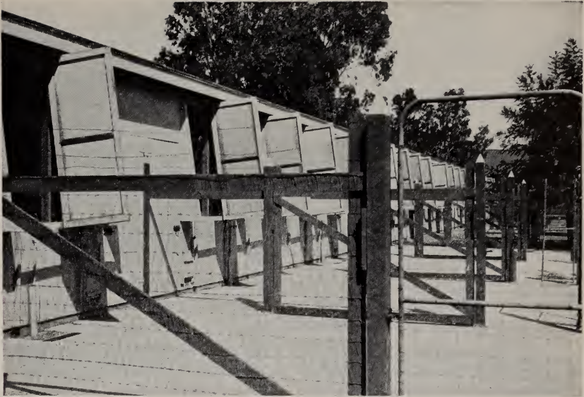
Fig. 63. A long laying house with concrete yards. Note the board-covered drainage pit next to the house which receives waste water from drinking vessels through a vertical 2-inch rain conductor pipe.
